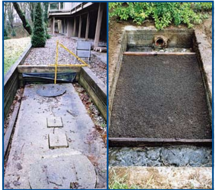
Figure 4. Newer style septic tank
